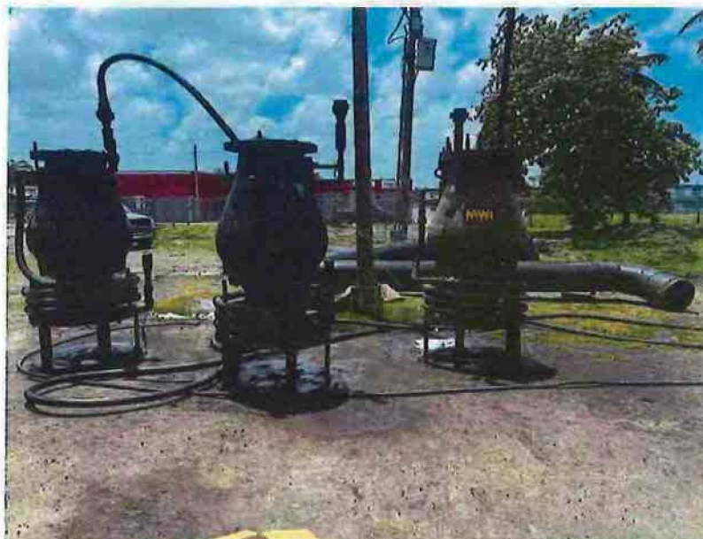
Performance Test Being Conducted at Sabana Pump Station
